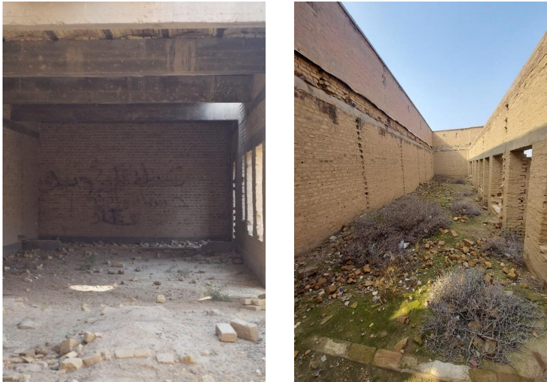
Fig. 5: left: rooms in the northeast section. Right: rooms in the southwest section (researcher)
